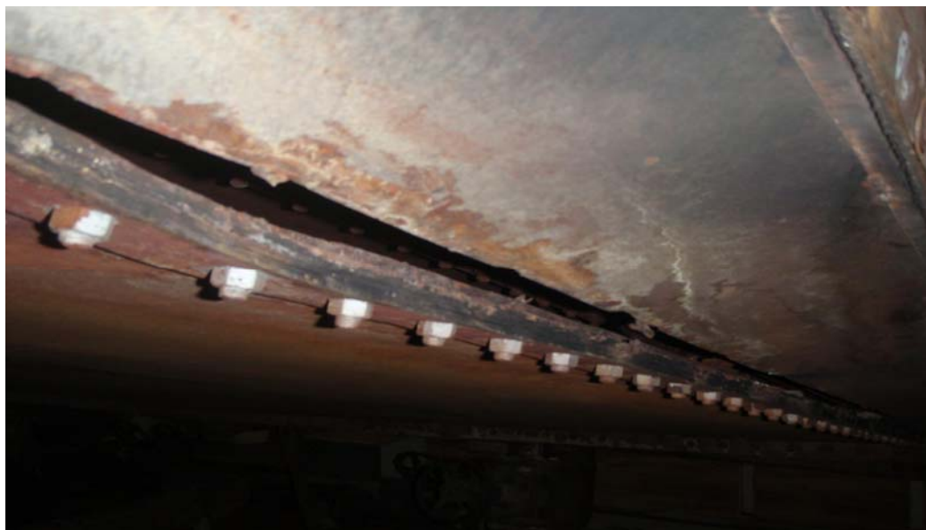
The picture shows furnace casing damage
