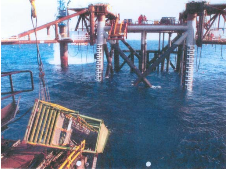
The gangway collapsed into the sea
