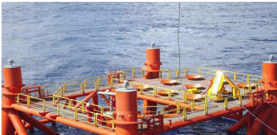
Platform jacket showing personnel lifting device and crane wire.
