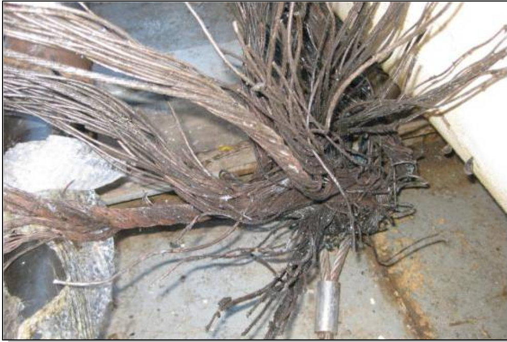
Photo from a recent incident on a facility in Australian waters
