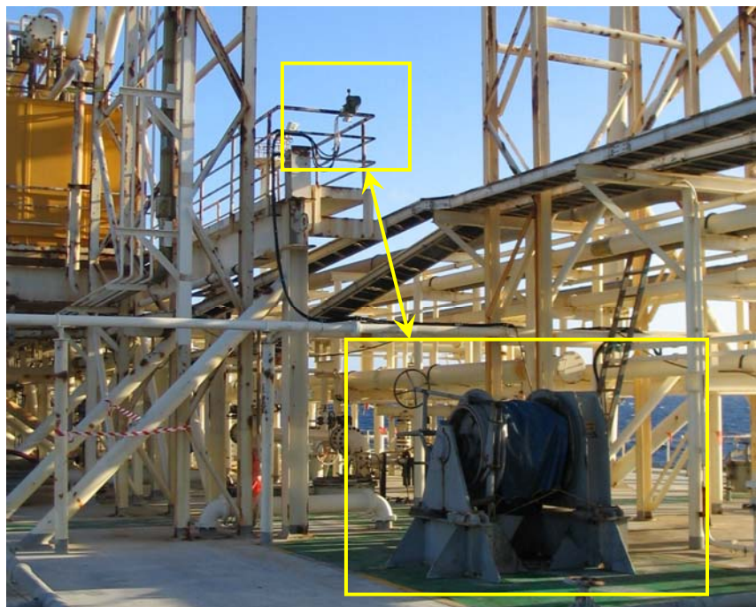
Operating station has been moved away from the winch to a safer location.
