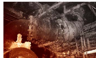
Aftermath of engine room fire (Alert 17, NOPSA website)
