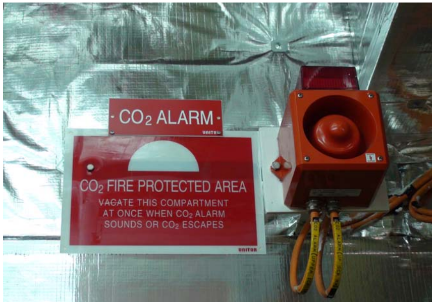
This is a good example of signage and an audio visual alarm on an older facility
