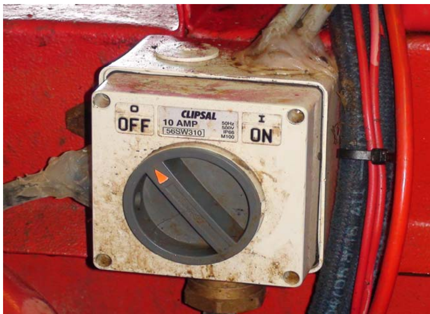
This is an example of incorrectly glanded cables entering this isolator located in a zone 2 hazardous area. In particular note the use of silicone to seal the cable entry.
