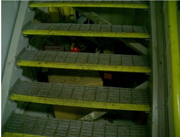
Combustibles such as cardboard under escape stairs to temporary refuge (TR) could pose a fire hazard and impair evacuation
