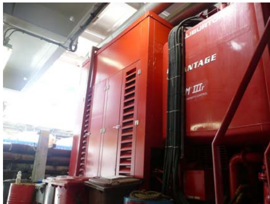
An acoustic enclosure fitted to a cementing system contributes to effective noise management.
